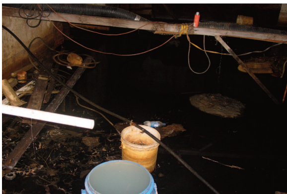
Figure 3. Basement with standing water and debris.
