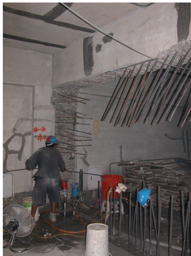
Fig. 1. The workplace of these workers was in the basement, which was more than 10 meters underground with high temperature, high humidity, and poor ventilation.
