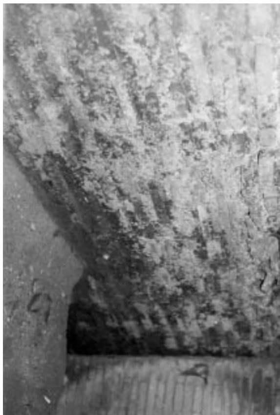
Figure 2. Type of deterioration: whitish efflorescence.
